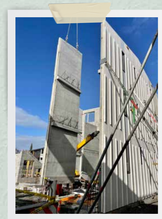
Image: Progress at Bader Ventura as off-site manufactured panels with windows installed are craned into place
